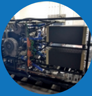
FUEL CELL MODULES / RACKS
